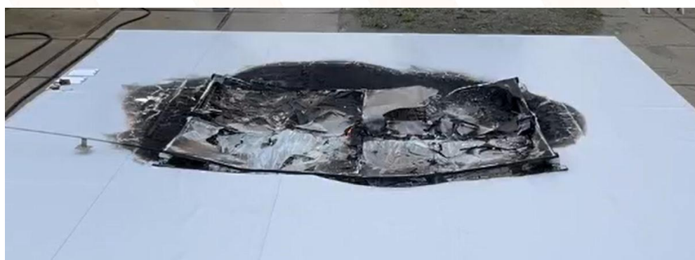
Figure 5: Flat roof with EPS foam and a maximum overlap of glass fleece installation – damage demonstrates the effectiveness of the glass fleece and minimal fire spread underneath the completely destroyed PV system.
