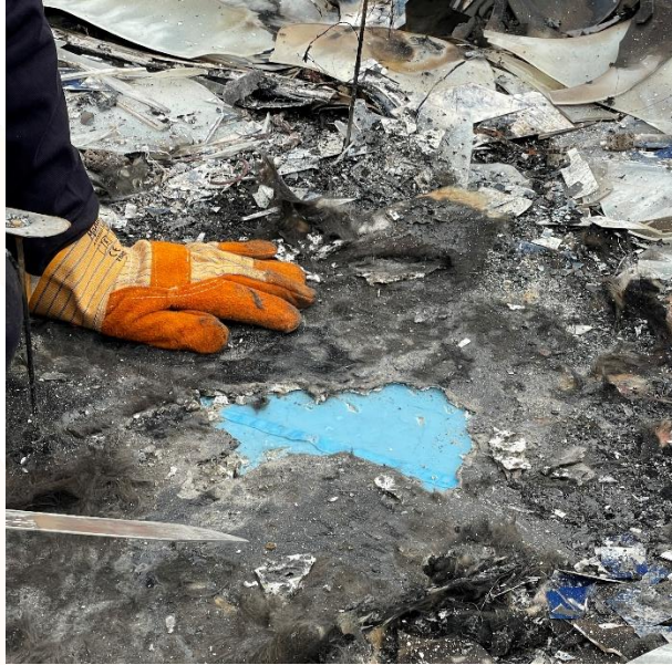
Figure 6: Once the glass fleece and melted EPS insulation residues were removed, the undamaged vapour barrier (blue) on the cement-bonded particleboard was revealed.
