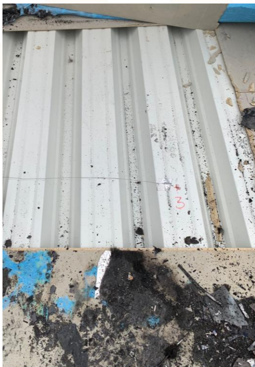
Figure 7: Beneath the undamaged cement-bonded particleboard, the trapezoidal sheet deck is also intact. No burn-through of the trapezoidal sheet occurred.
